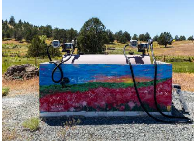
Diesel - Unleaded split tank; 275 gallons each side
