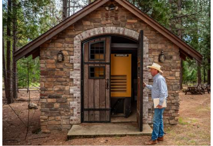
Caterpillar 70kW Electrical Emergency Generator
